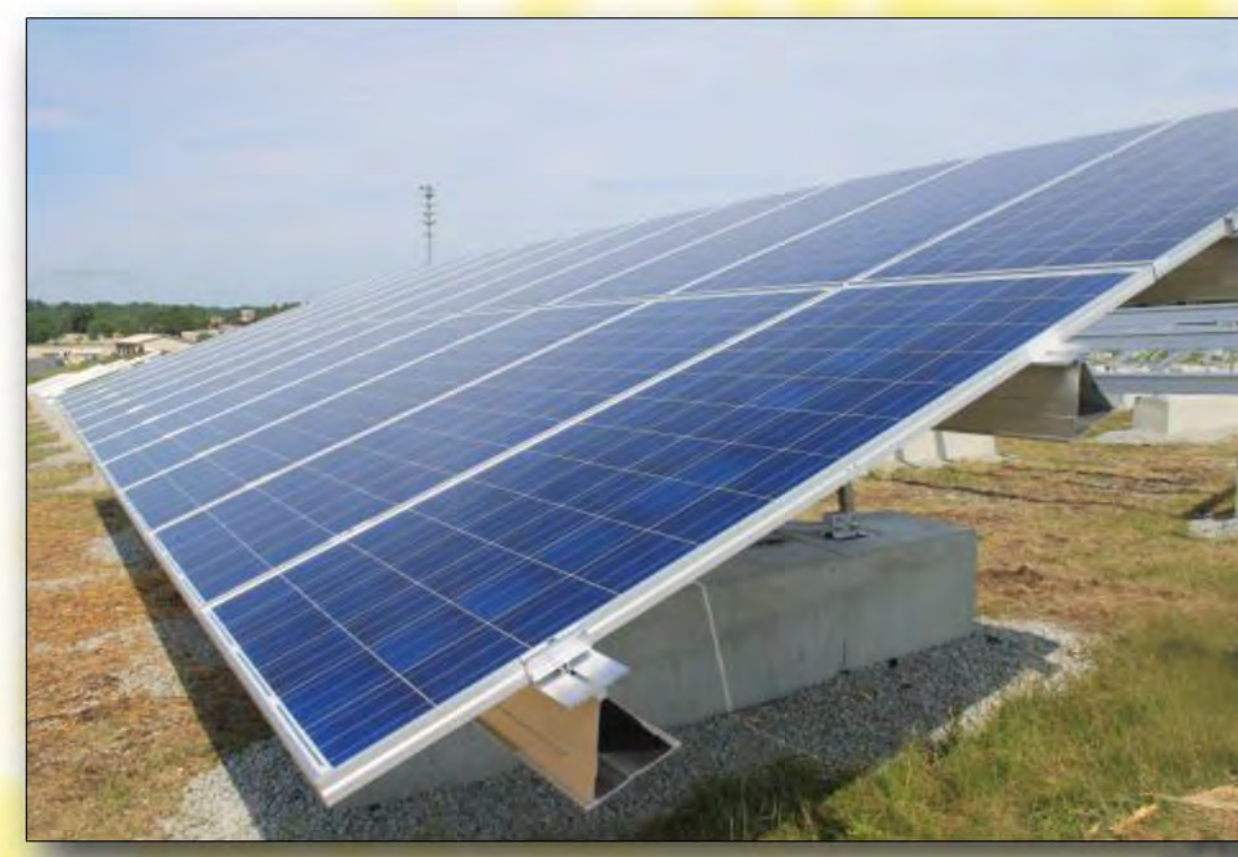
With Ballasted Solar and Back-up Power
