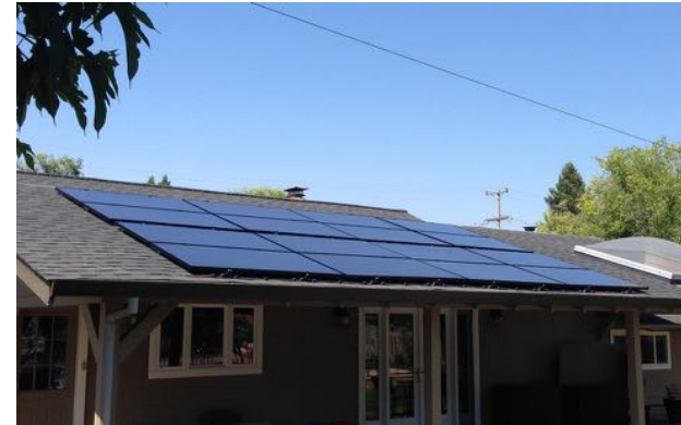
Solar photovoltaic (PV) panels
